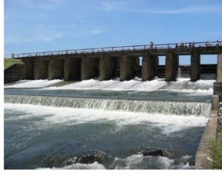
Ten spill Doors of Samudraya
