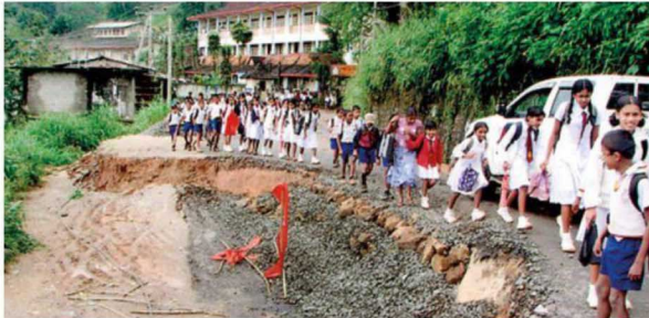
February 2011: The road close to Sri Sumangala Vidyalaya caved in due to heavy rains
