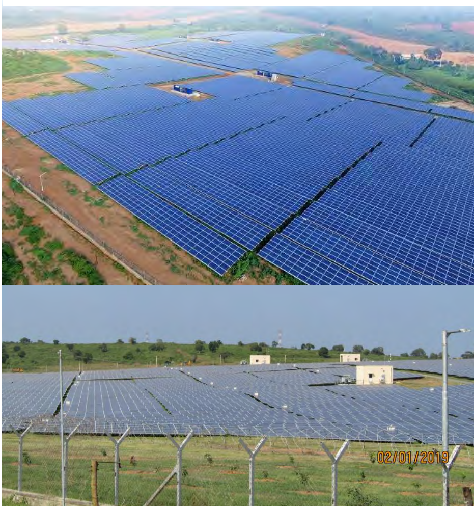
Figure 5-5: Solar Power Park - Burutankanda
