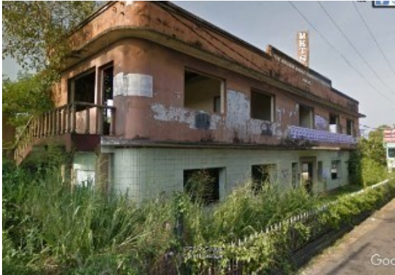
Degraded buildings at Pettigalawatta
