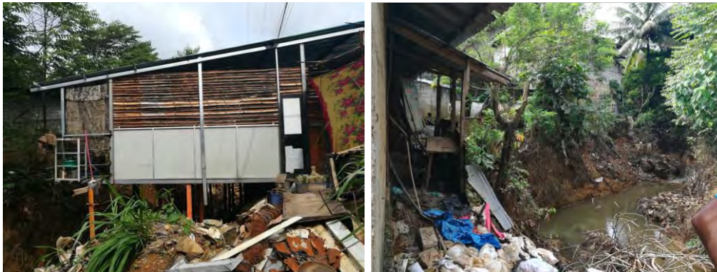
Figure 5.20 Sambawela Canal Reservations Encroachments
