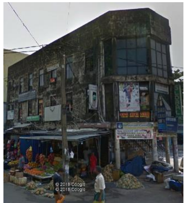
Dilapidated building at Sea Street
