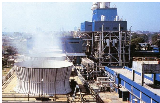
Figure 46: Kelanitissa Power Plant Image Courtesy: Intsnl.com
