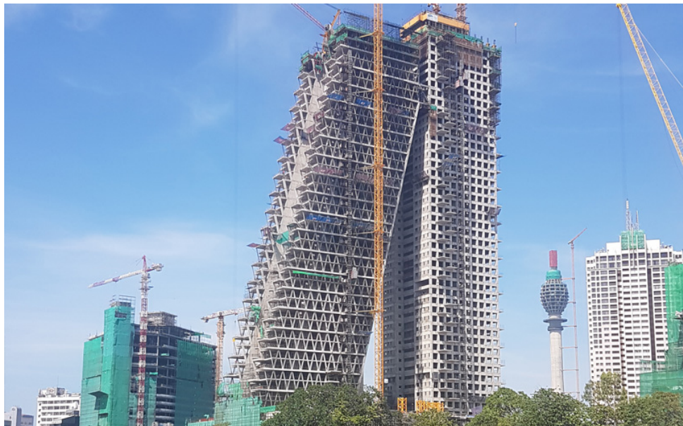
Figure 150: Altair Building (Mixed Development) located at Gangaramaya, Colombo in Construction Image Courtesy: skyscrapercity.co
