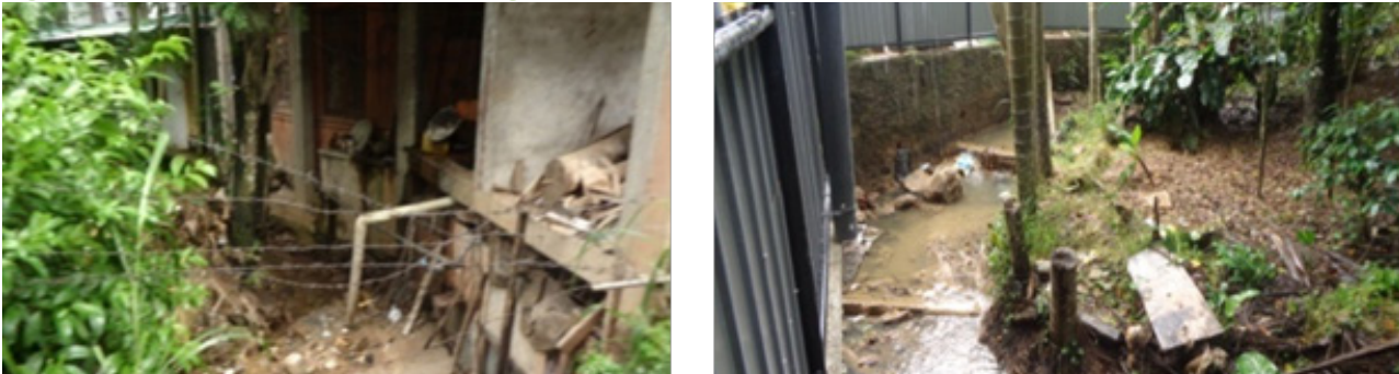
Figure No 5.11: Waste water discharge in to the natural channels from restaurants in Ella.
