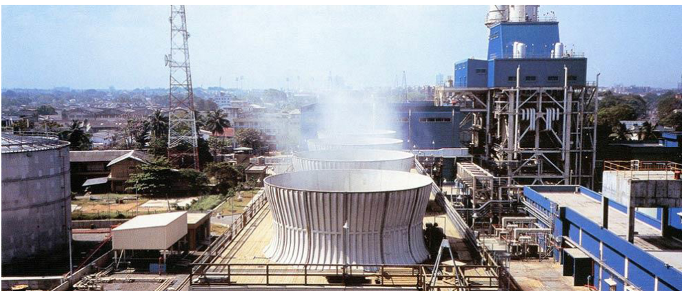
Figure 46: Kelanitissa Power Plant Image Courtesy: lntsnl.com
