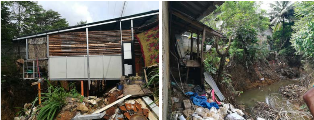
Figure 5.20 Sambawela Canal Reservations Encroachments Source: Captured by Udari Hettiarachchi, 2018/06/21
